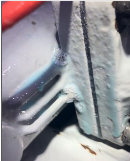
Figure 1: External leak through stitch weld
